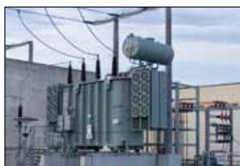
real image of a transformer
