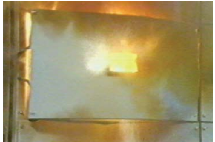
Steel panel being ripped from its hinges and bolts during an arc blast in an enclosure with no arc resistance mechanisms. Note the hole blown through the solid steel panel.
