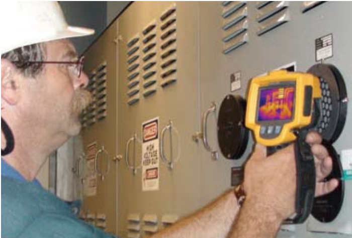
Example of a thermographer using an IR window and wearing standard level of PPE required while operating energized electrical equipment in an enclosed and guarded condition.
